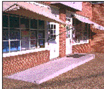
The awning and awning support over the walk to the entrance is too close to the ground and is a barrier to people who are blind or visually impaired.
